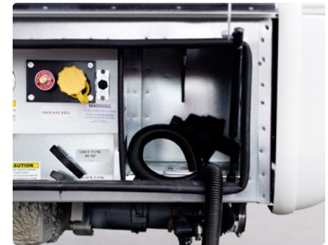
Macerator Sewage Discharge With Manual Disconnect
